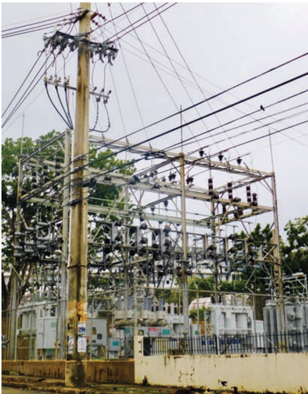
PREPA's substation in Hato Rey, San Juan, Puerto Rico.
