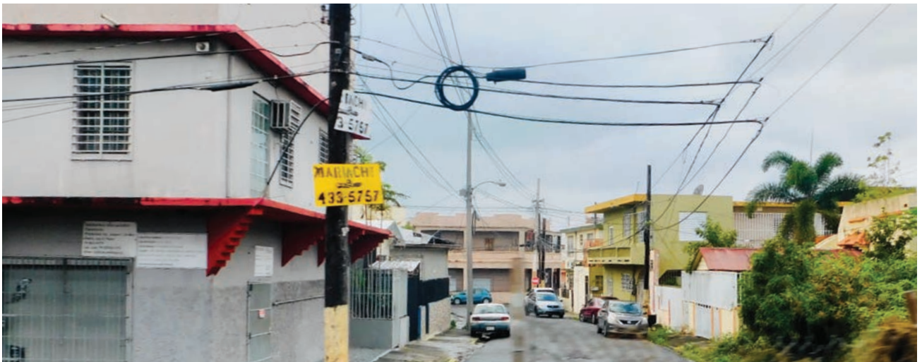
Current state of poles and wires part of the PREPA's distribution system. Santurce, San Juan, Puerto Rico.
